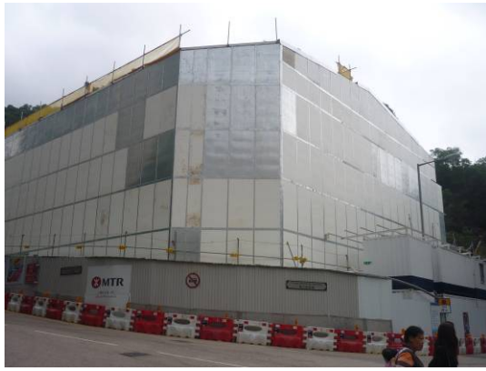
Photo 1: Noise enclosure in Sheung Mun
