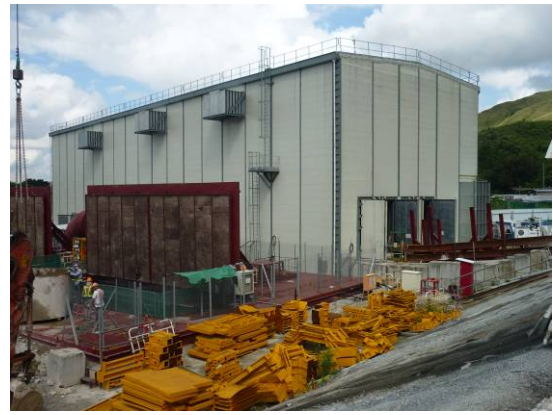
Photo 2: Noise enclosure at Tai Ko Po
